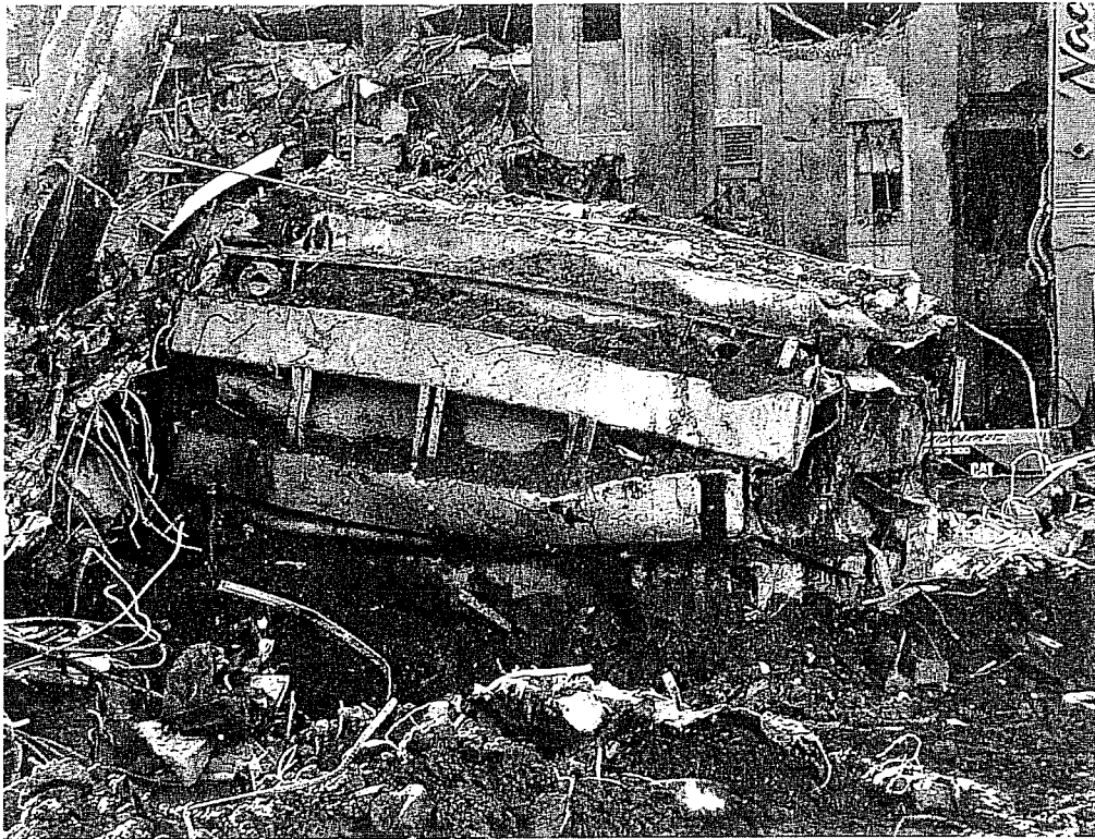
FIGURE 16.1 A 65 MVA, 138/13 KV transformer crushed when the World Trade Center collapsed. (From ConEd-ison, New York, NY. With permission.)
